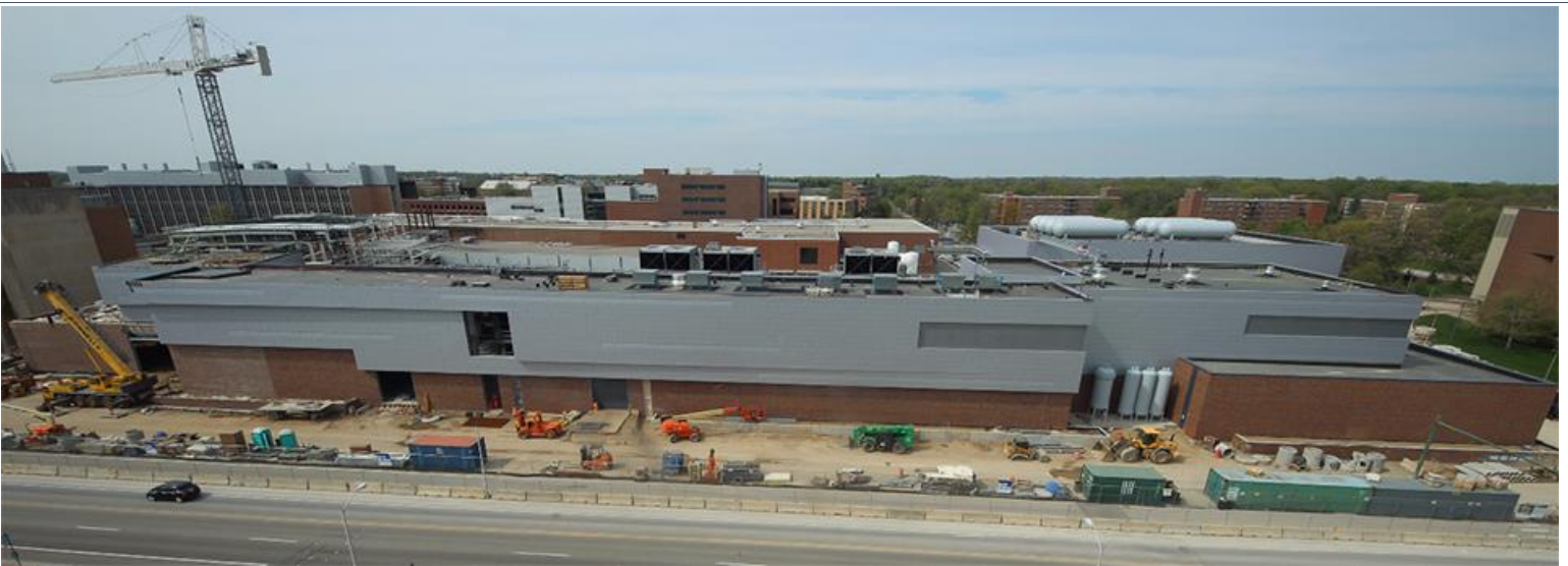
Figure 3 This is a camera view from the south showing the FRIB construction area from a camera located at MSU's Molecular Plant Sciences Building.
